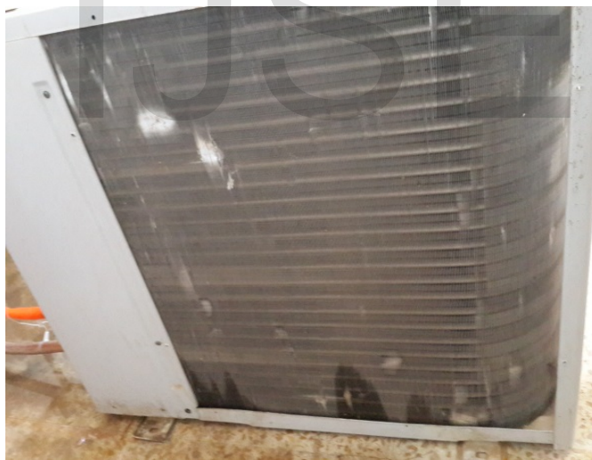
Figure (5) outdoor unit
